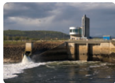
Figure 5 The Annapolis tidal plant, in Nova Scotia, is North America's only tidal plant. It produces up to 20 MW of power daily.
