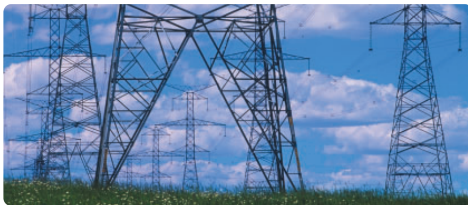
Figure 1 High voltage transmission lines carry electrical energy from power generating stations.
